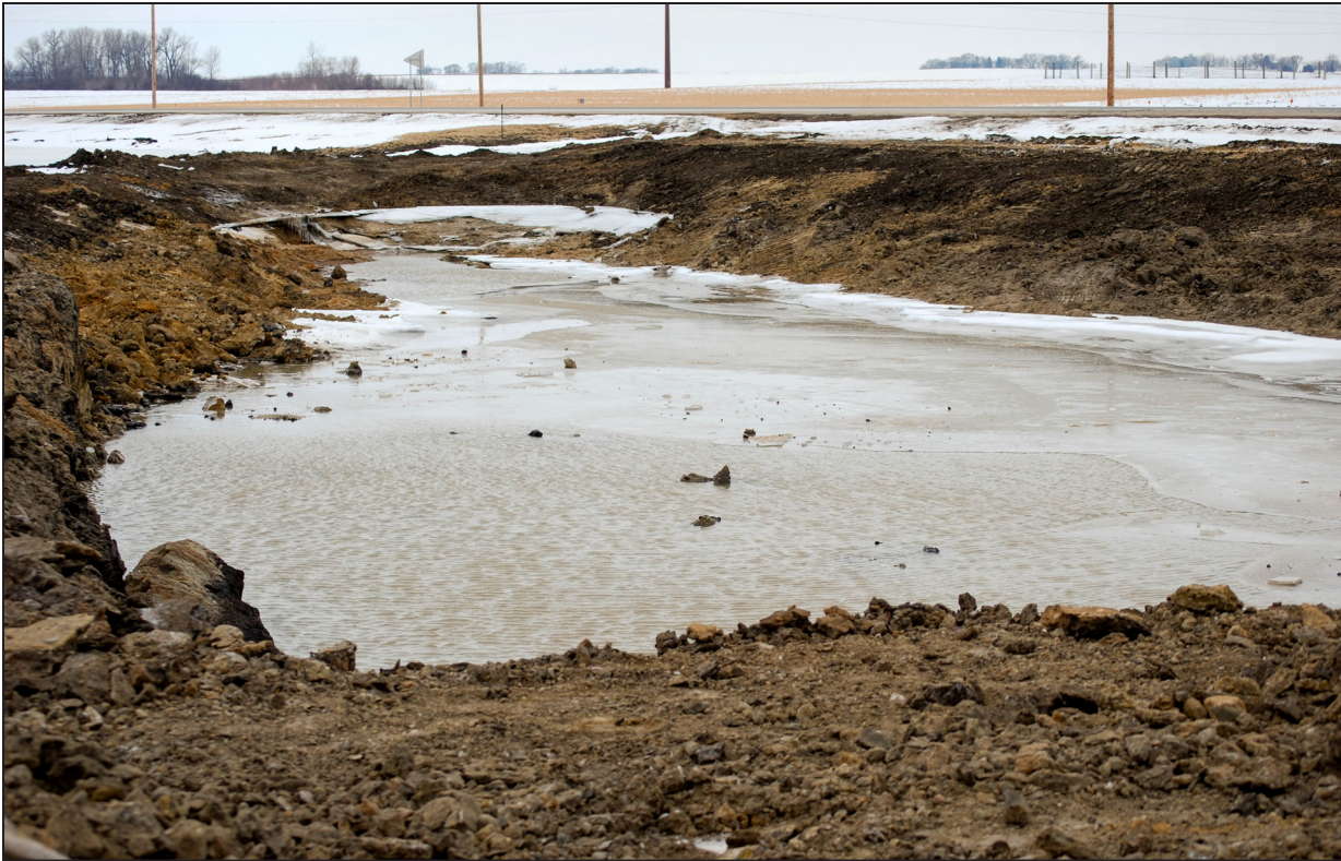
A tributary to the South Branch Vermillion River will be diverted around a constructed wetland in Castle Rock Township while the plants take hold. The experimental nitrate treatment is slated to go online in 2019. Final ground work is scheduled for this spring. Photo Credit: BWSR
