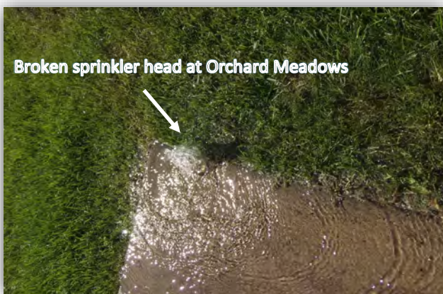
Broken sprinkler head at Orchard Meadows A broken sprinkler head can waste thousands of gallons of water per week.
